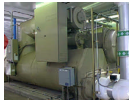
Figure 9. A typical chiller.
